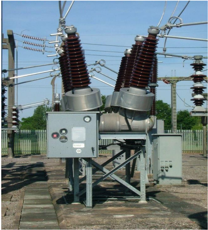
132 Dead Tank Circuit Breaker
