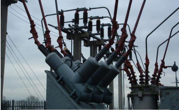
33kV outdoor Circuit Breaker
